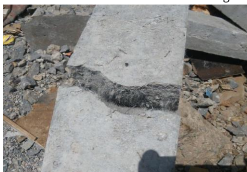
Figure: 6 Failure Pattern Observed In Beam
