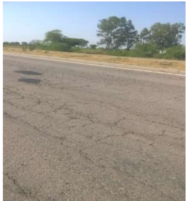
Figure-4 Alligator crack
