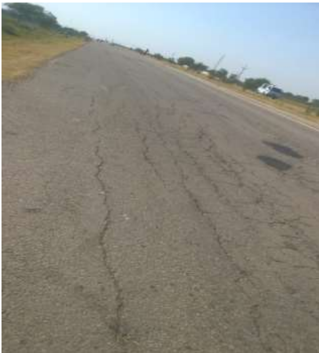
Figure-3 longitudinal crack
