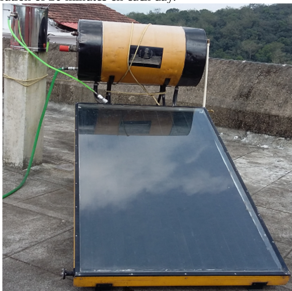
Figure 2. Liquid FPC installation on the roof top of Research Square building at Amal Jyothi College of Engineering, Kanjirapally
