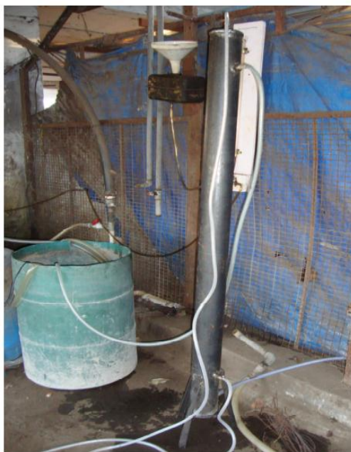
Fig 1 Water Scrubbing Unit
